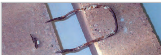
The majority of wall tie corrosion occurs within the bed joints of the external leaf
