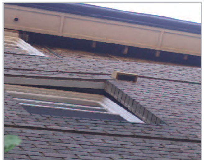
Bowed brickwork is a strong indicator of wall tie failure
