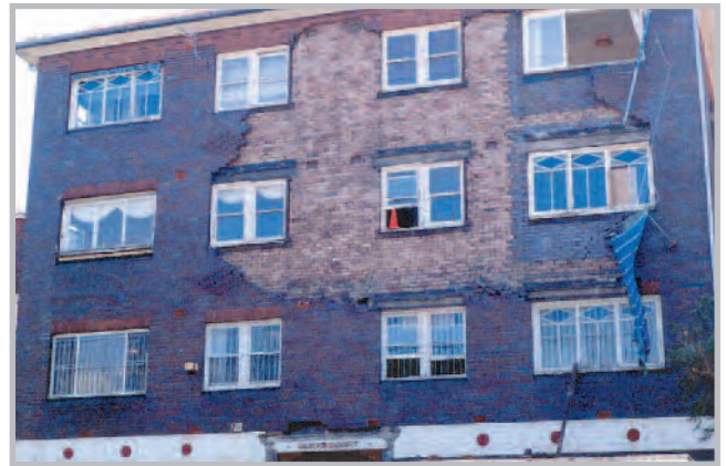
Brickwork collapse from a residential apartment block in Sydney, resulting from wall tie failure
