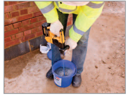
3. Stir thoroughly using a power-driven paddle mixer. Do not attempt to mix by hand as this will result in inadequate mixing
