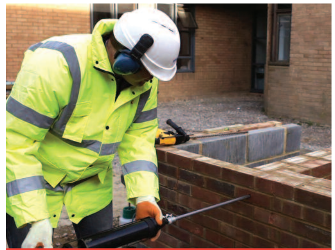
Inserting the grout-filled pinning nozzle, containing the CemTie, into the clearance hole
