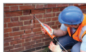
6. Inject CrackBond TE3 into the crack leaving enough space for making it good. Re-point the bed joints with matching mortar and make good the crack.
