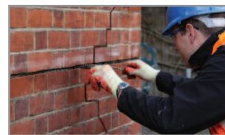
4. Using the HeliBar Insertion Tool push one HeliBar into the grout to obtain good coverage
